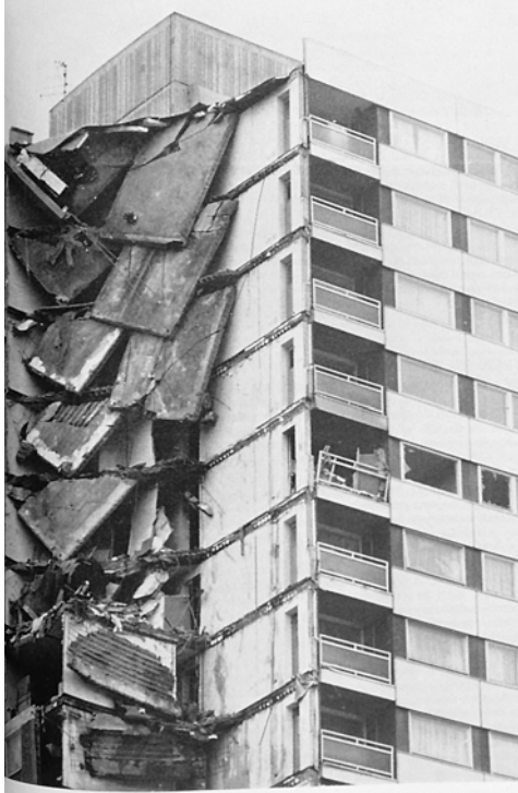
1.19 Architects' Journal (1968): Close-up of the collapse of Ronan Point tower block, Newham, London.
